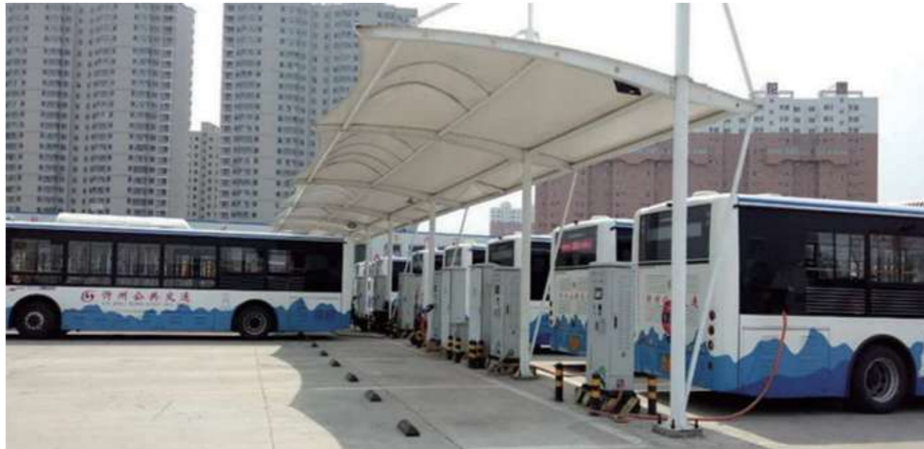
Xinzhou Bus Charging Station
