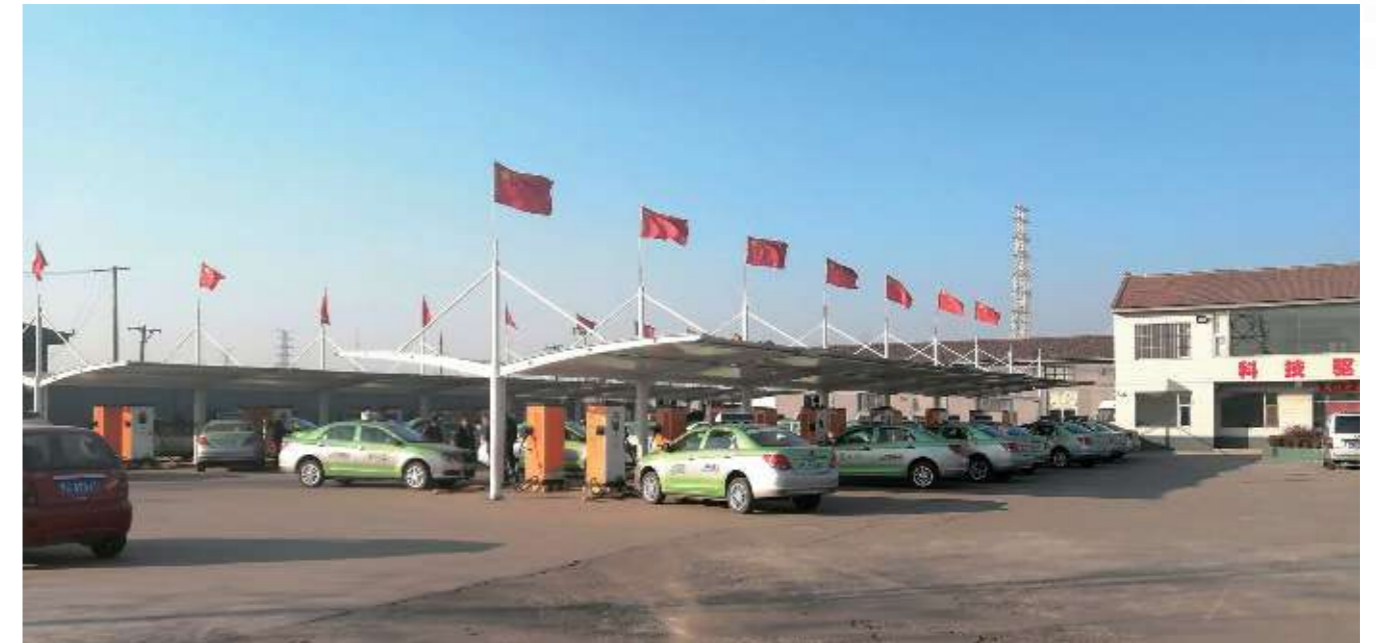
A public charging station in Yangquan, Shanxi
